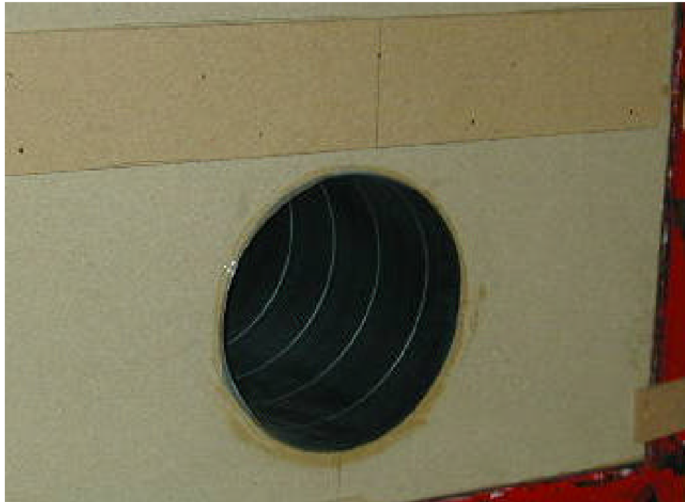
Photo B3: Outlet to Reverberation Test Chamber
