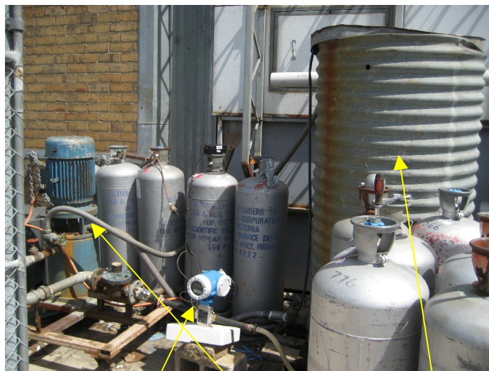
Figure 1 – Flow meter, high volume pump and water tank
