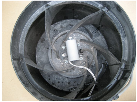
Figure 6 – Sample 2, The Engineer noted minimal water near fan motor enclosure, no water inside fan motor
